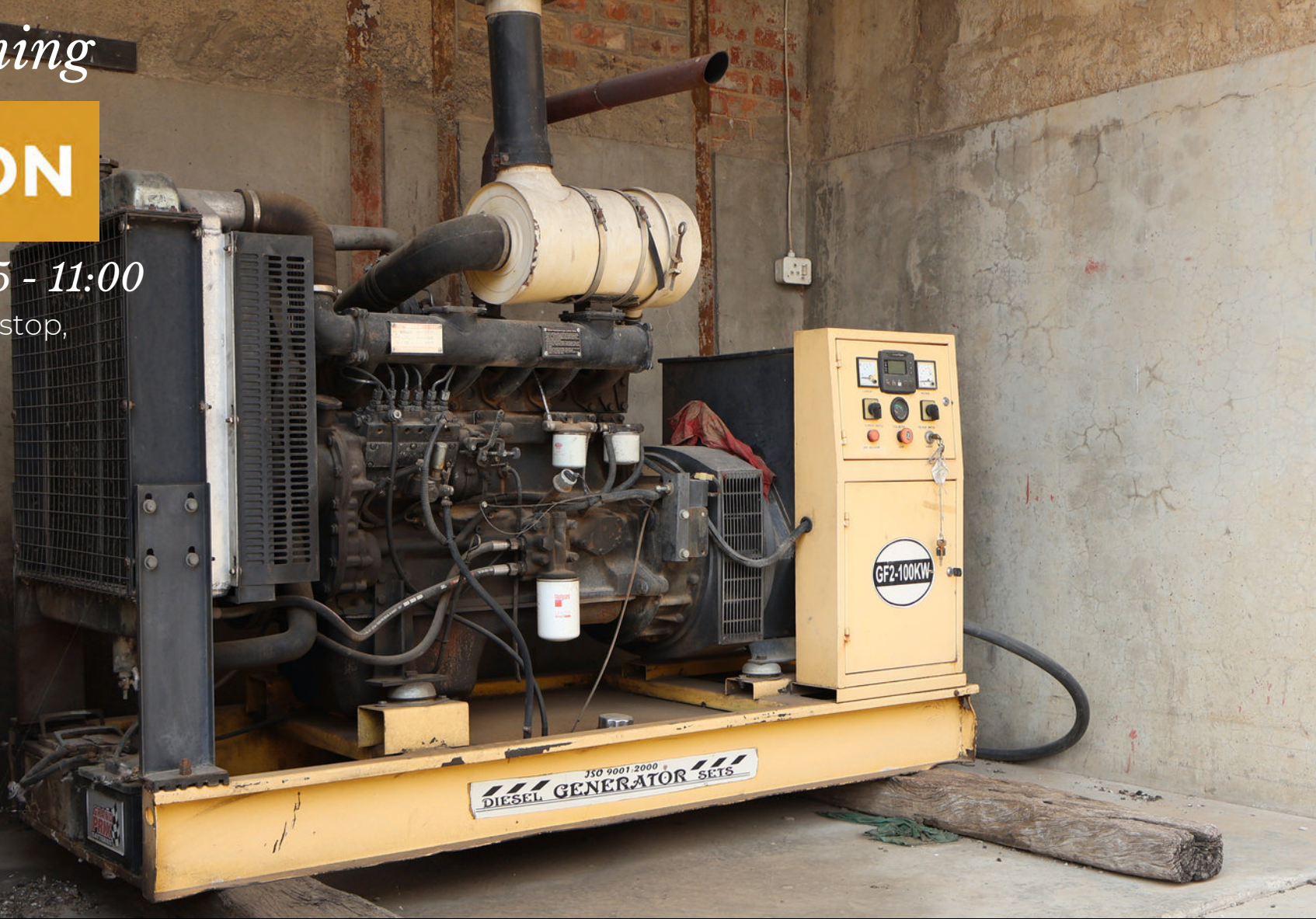
Diesel Kragopwekker 100kva
